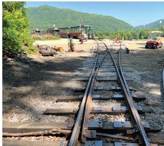
Switch outside tunnel 2 for the connector track from the new loop. Photo courtesy Curtis Brookshire.
